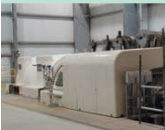
Electricity is generated at three of our pulp and paper mills.
